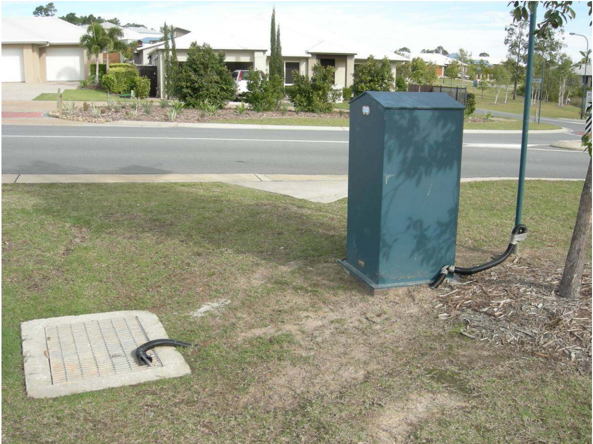
Figure 1: Monitoring station installed in a swale at Coomera Waters, Qld
