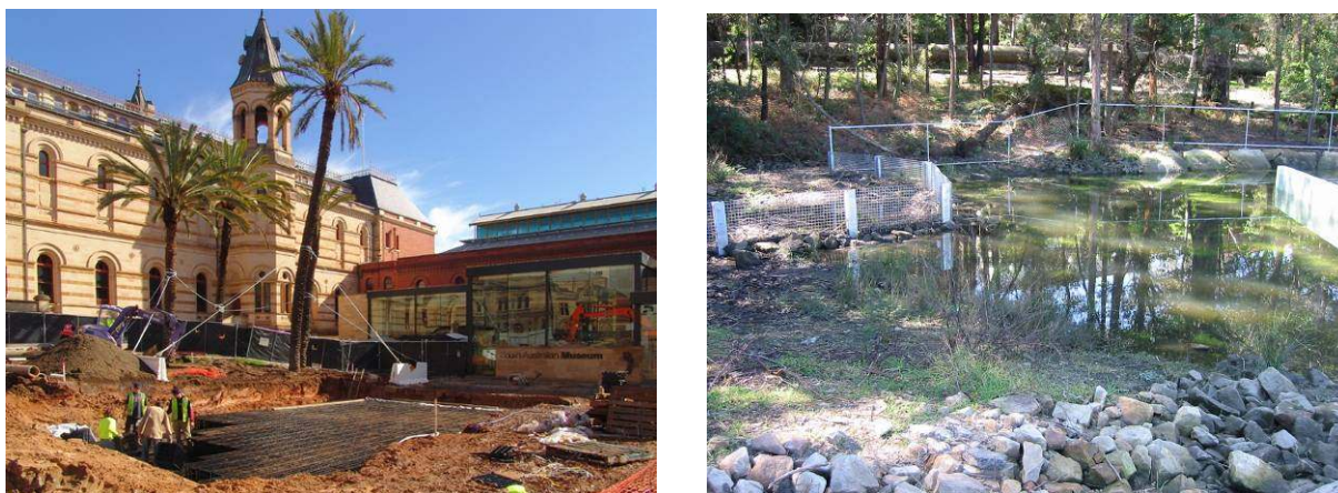
Figure 3: Stormwater storage being installed at the South Australian Museum (left), and stormwater harvesting pond at Barra Brui oval, St Ives (right)
